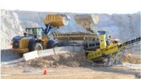
Conveyer Belt to On-site Wet Plant
