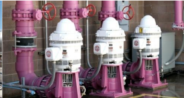
Automated Asset Management
