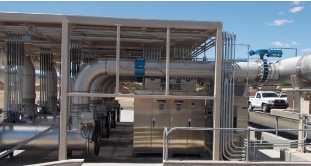
Advanced Treatment Systems
