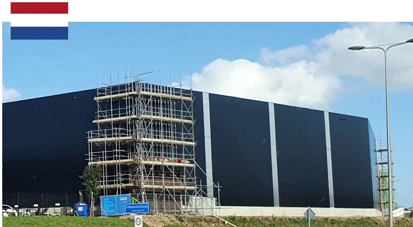
Satellogic High Throughput Plant, Netherlands
