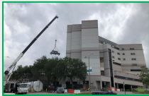
Mechanical Infrastructure Projects
