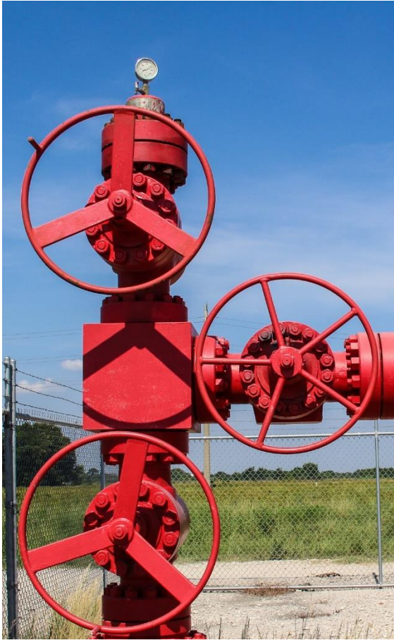
Natural gas storage wellhead, Houston, Texas
