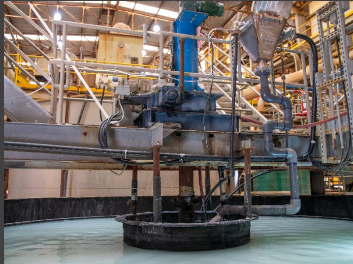
Monazite "crack-and-leach" equipment at Energy Fuels' White Mesa Mill
